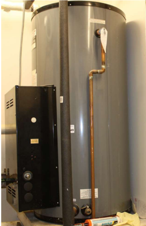
Figure 3 Electric Water Heater
