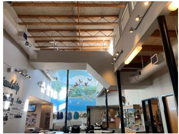
Figure 11: Lobby Track Lighting
