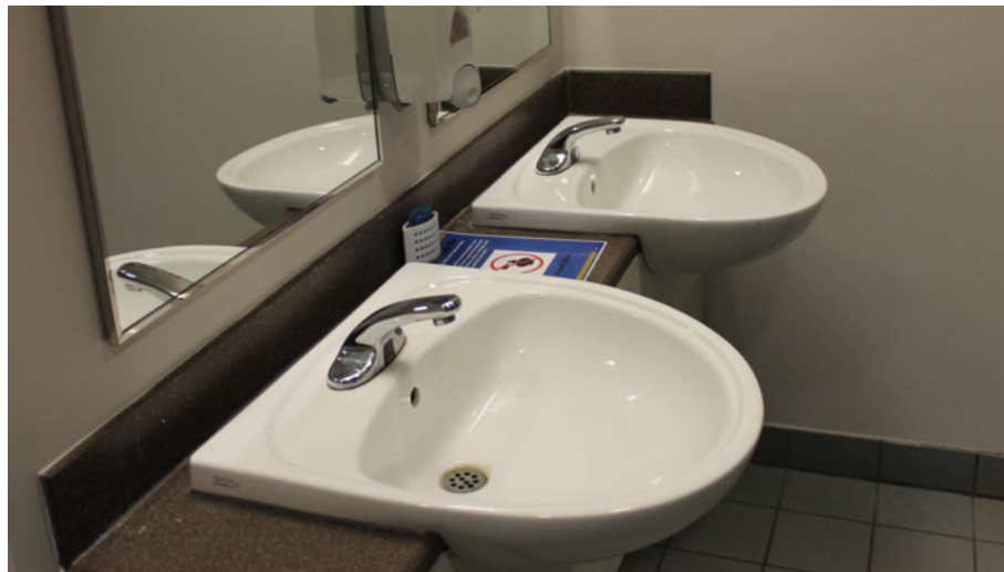
Figure 5 Touchless sinks in men's washroom
