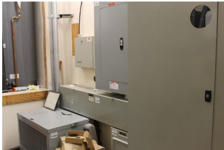
Figure 3: Main 600V Splitter and panels
