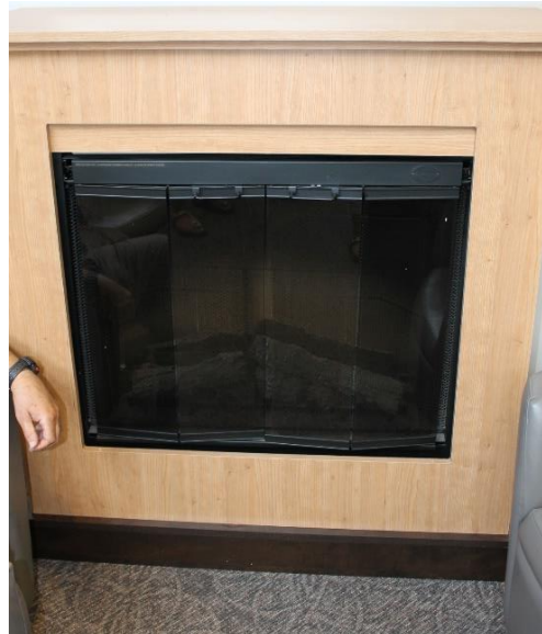
Figure 7: Existing Electric Fireplace
