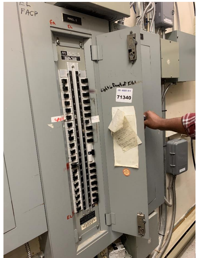
Figure 5: Branch Circuit Panelboard
