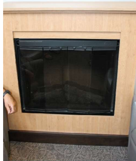
Figure 15 Electric Fireplace in Lounge Area
