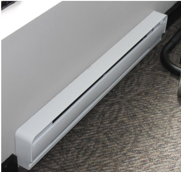
Figure 6: Existing Baseboard Heater
