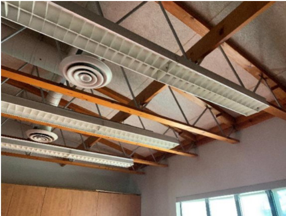
Figure 10: Multipurpose Room Lighting
