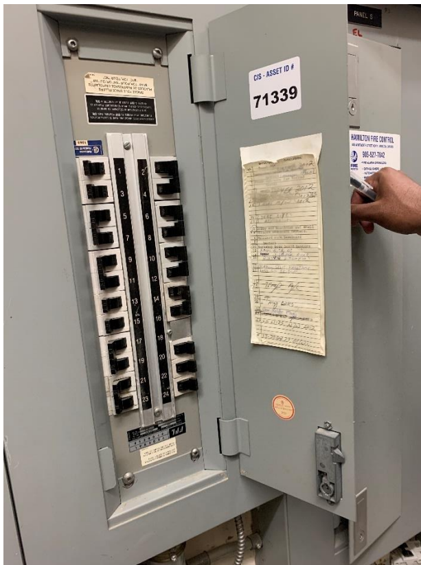
Figure 4: Branch Circuit Panelboard
