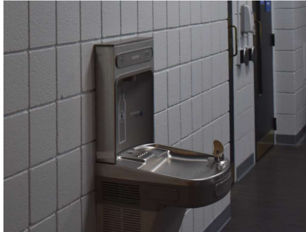
Figure 6 Typical Water Fountain in Facility
